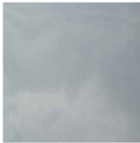
Weathered Concrete Ref: 92
